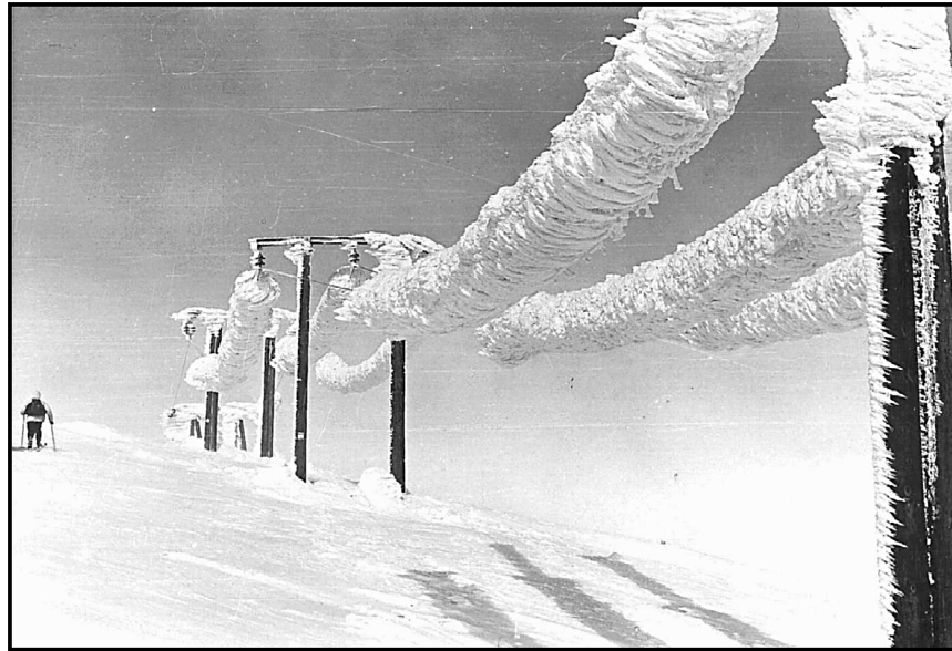
Figure 1. Rime on a 22 kV overhead line in Voss, Norway, 18 April 1961. This event is the highest iceload recorded on power lines in the world: 305 \text{ kg m}^{-1} on each span (photograph from Olav Wist).
