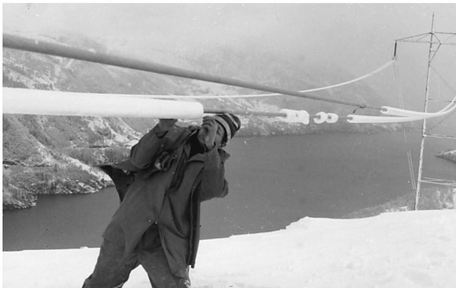
Figure 4. Wet-snow accretion on a 300 kV power line in Dale-Fana, Norway (photograph from Satnett).
